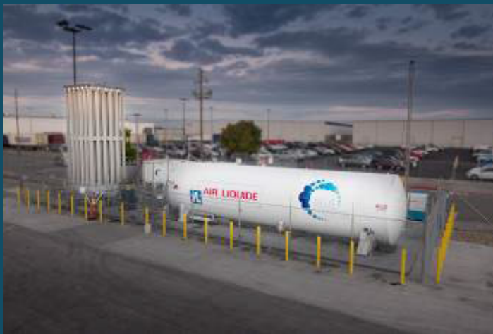
Figure 10: Liquid Hydrogen Storage by Air Liquide
