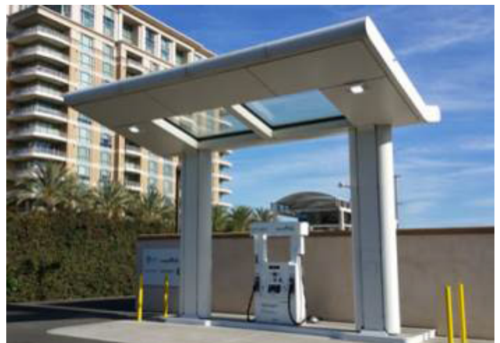
Figure 4: Hydrogen Refueling Station at UCI by Air Products
