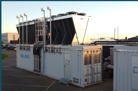
1MW decentralized power generation for EV charging
