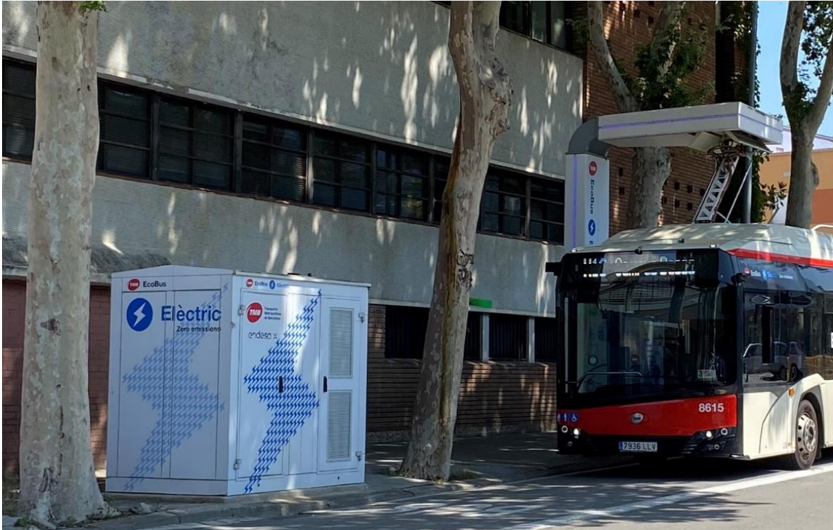
Figure 3 – Pantograph opportunity charging and infrastructure.
